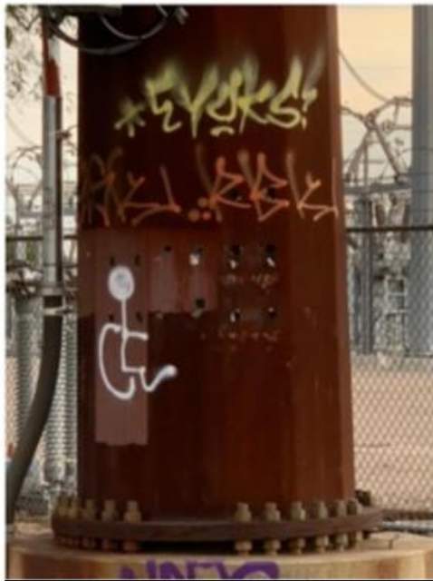
Fig. 5: TEP Pylon with Graffiti
